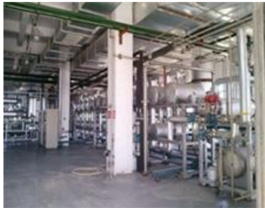
Figure 6-4: Photographs of compact zeolite membrane plants processing 1,000 to 3,000 gallons per day of wet ethanol [S24].
