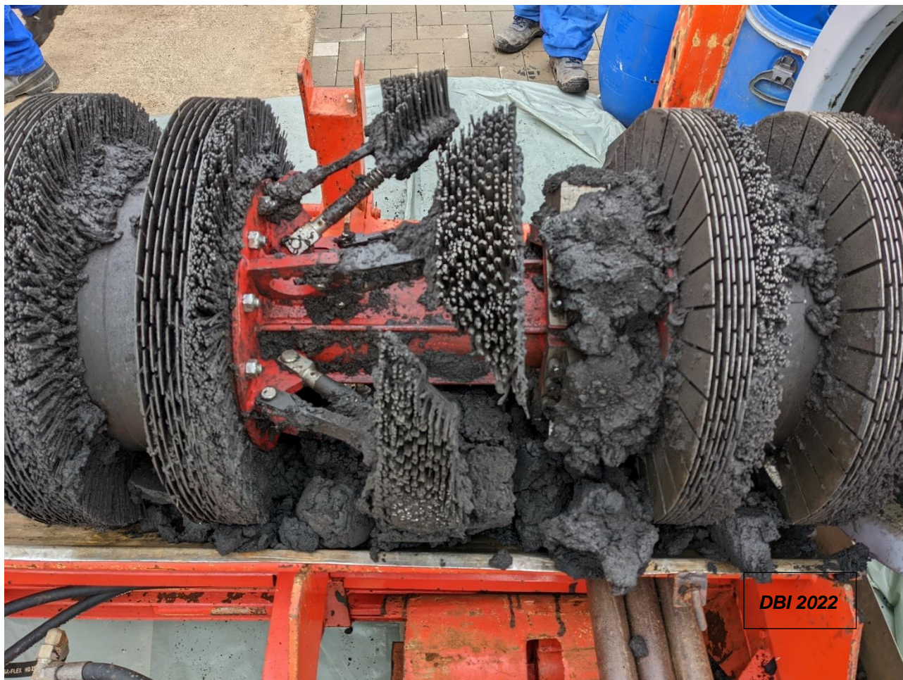
Figure 10: Deposits from a transport pipeline, second cleaning pigging
